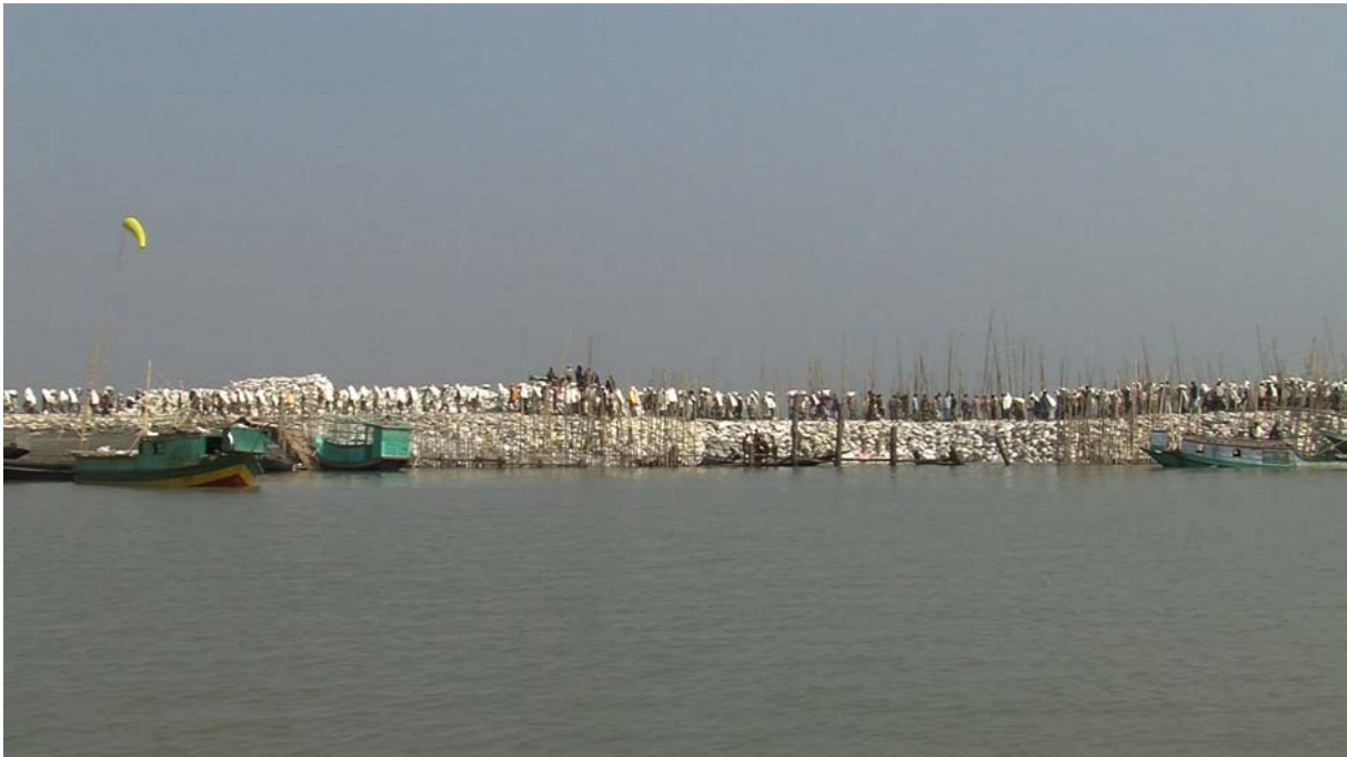
Fig 5. Deep Weather (2012) communal embankment building in the Bengal Delta.
